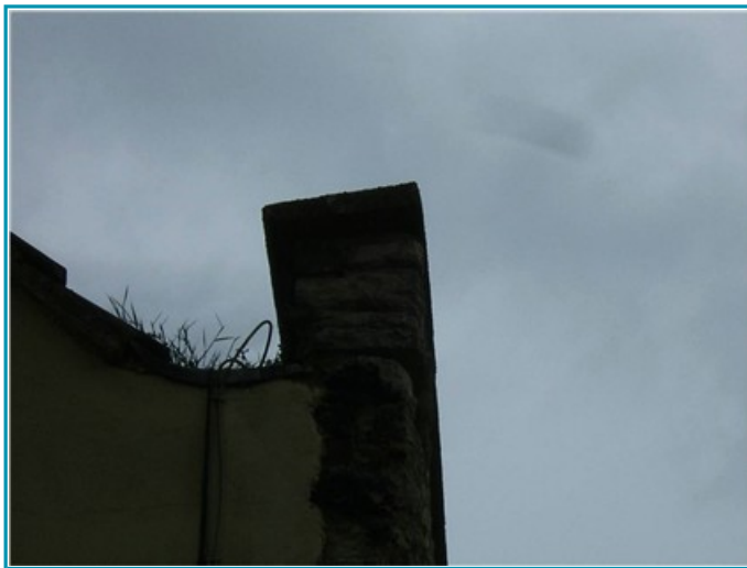
Blocked gutter behind parapet wall at front of property
