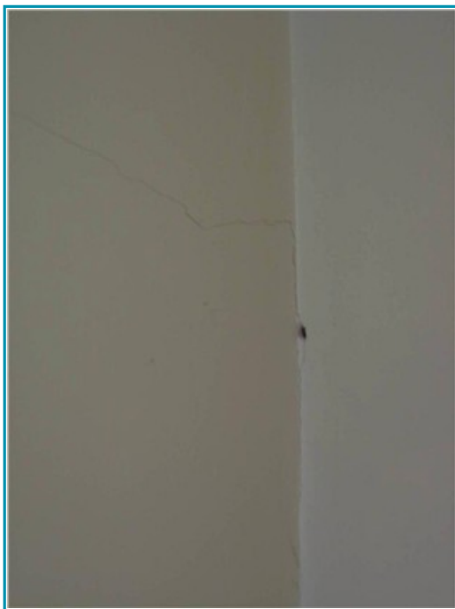
Cracking on internal wall
