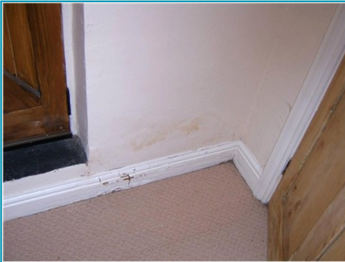
Rot in skirting board in rear reception room
