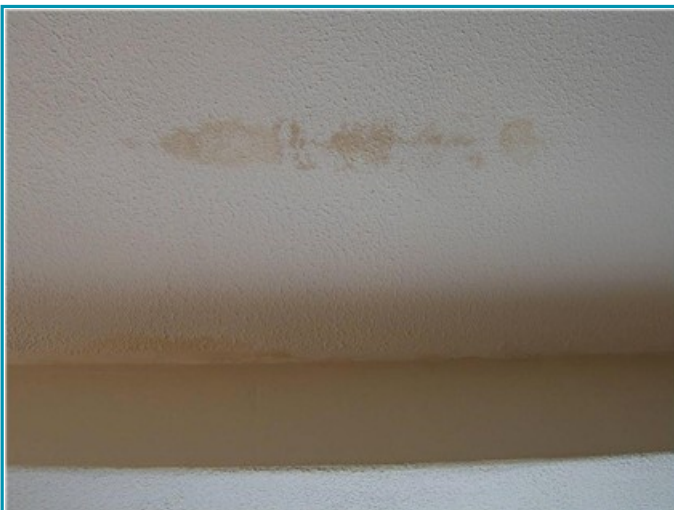
Damp on dining room ceiling
